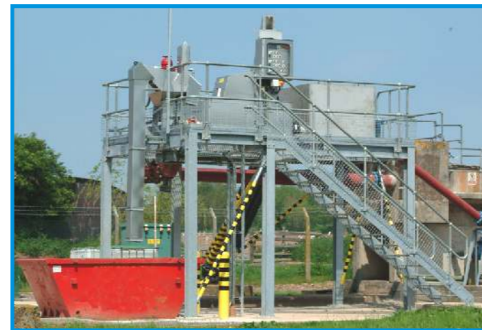
Screener in prefabricated inlet on tower
